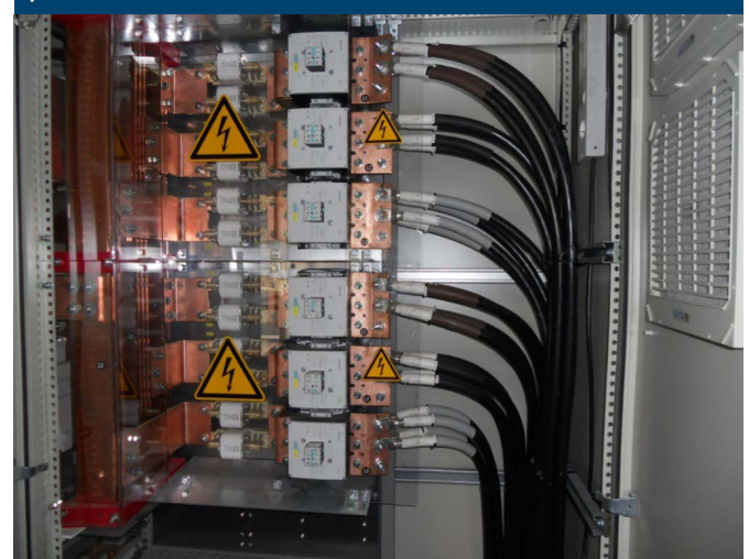
Fig. 8: Example of panel in machinery house with cable protection fuses
