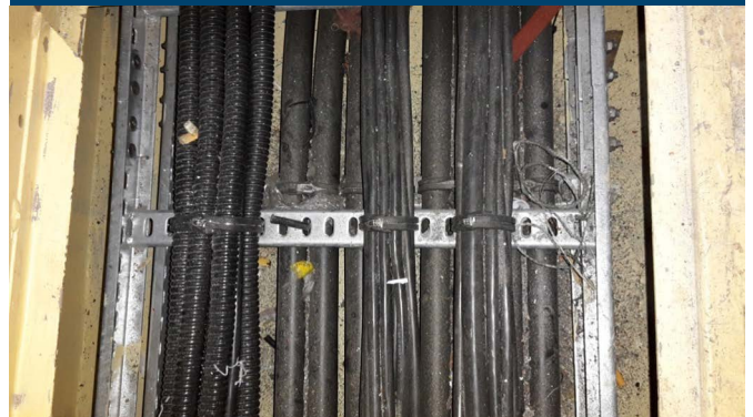
Fig. 6: Typical situation of cable routing under machinery house floor
